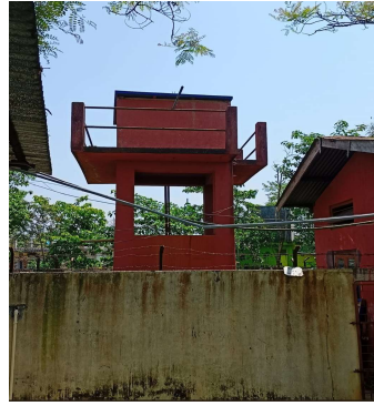
Photo.10: Water Storage Tank
