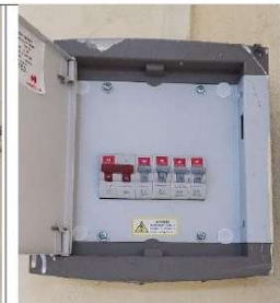
Photo: DB at Room #7: 1 x 40A DP Isolator (Main Incomer) 4 x 10A SP MCBs (Outgoing)
