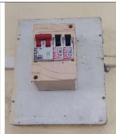
Photo: DB at Room #9: 1 x 40A DP Isolator (Main Incomer) 2 x 6A SP MCBs (Outgoing)
