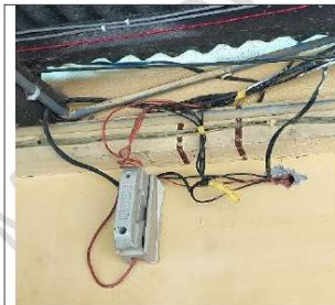
Photo: 100A Fuse at grid supply incomer
